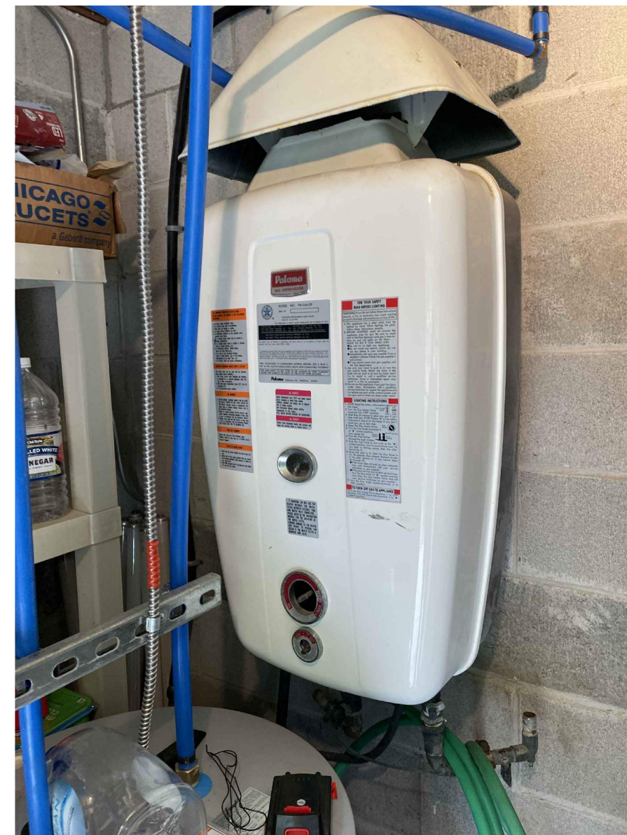
GAS HOT WATER HEATER
