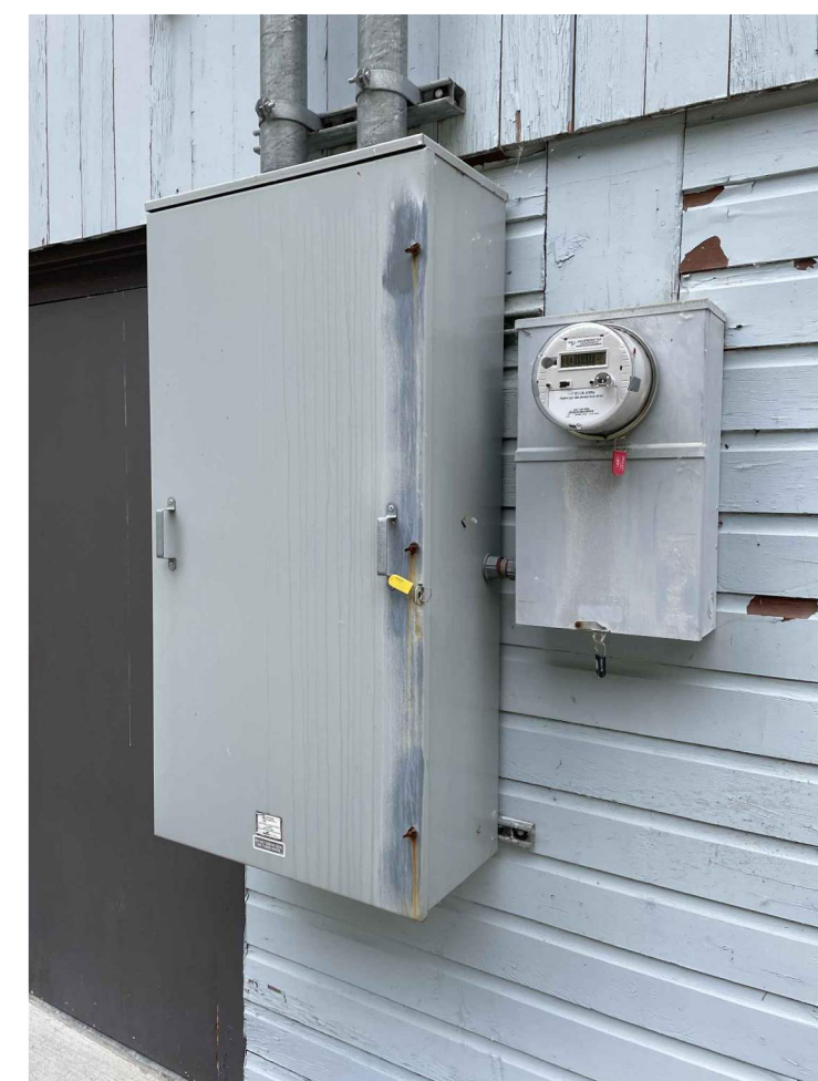
EXTERIOR ELECTRICAL MAIN DISCONNECT AND METER
